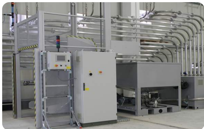
Thrust loading unit with Octabin station
