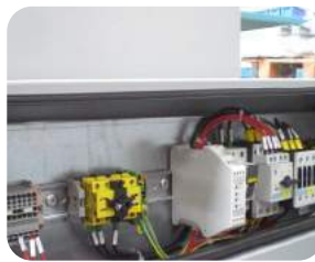
Safety control unit
